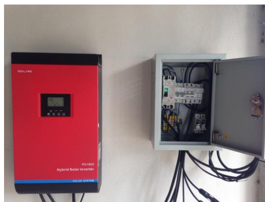
Figure 8 Inverter control system
