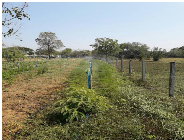
Figure 5 Sprinkler heads system for tilth
