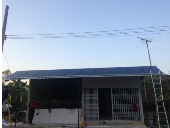
Figure 3 System of Roof Photovoltaic Array
