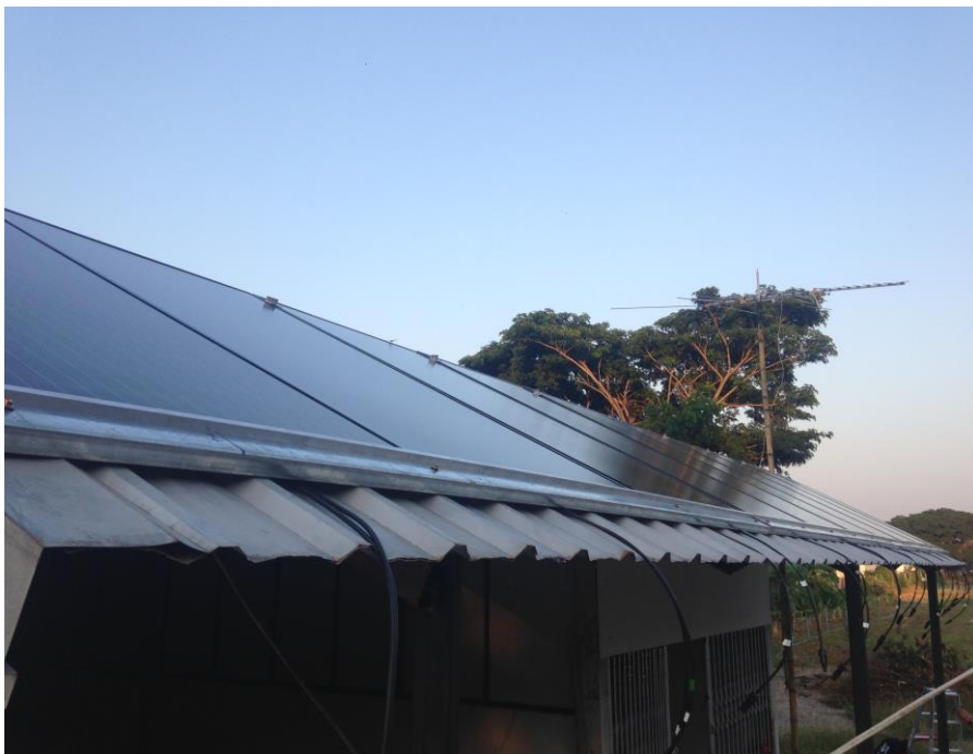
Figure 2 The Roof Photovoltaic Array
