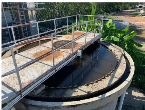
Figure 1: Activated sludge in KMUTT Bang Khun Thian
